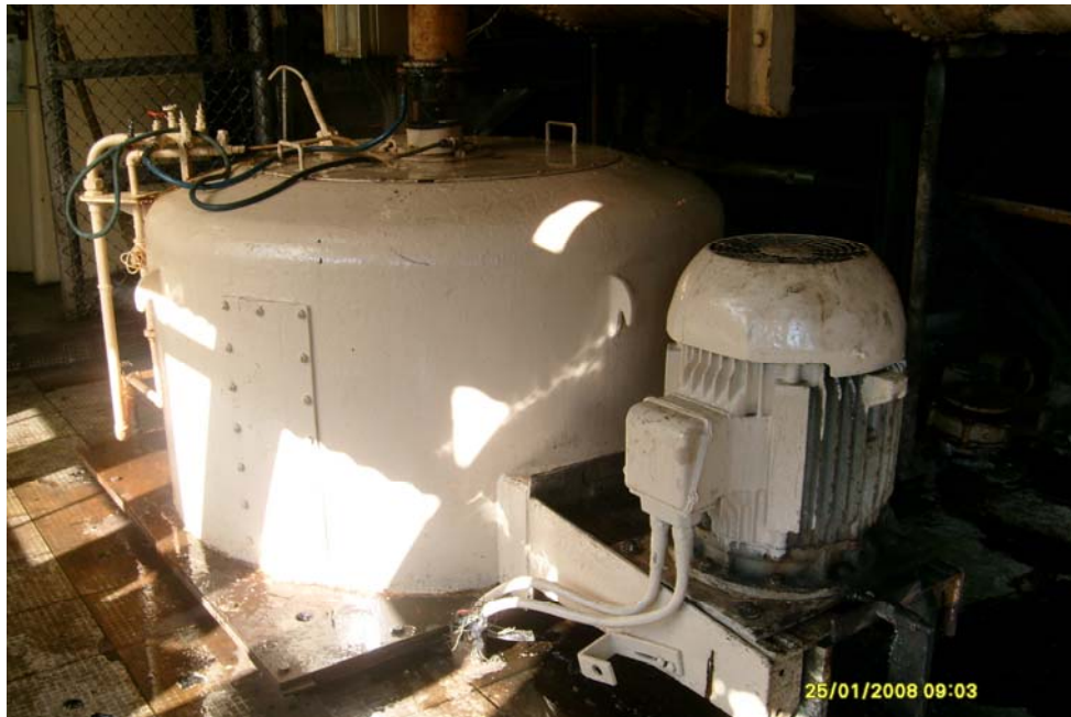
Fig. 1. Rota 900 High Grade continuous Centrifugal installed at Frome
